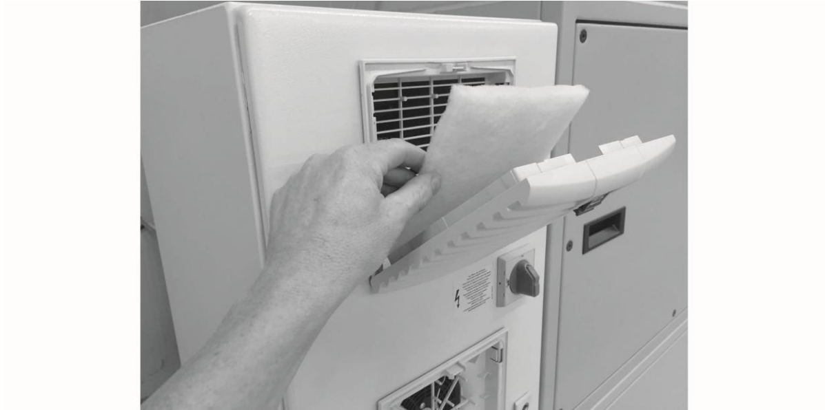
Fig. 39: Filter replacement in control cabinet
